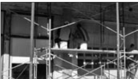
Weeks of painstaking labor to remove peeling paint layers from the East Façade
